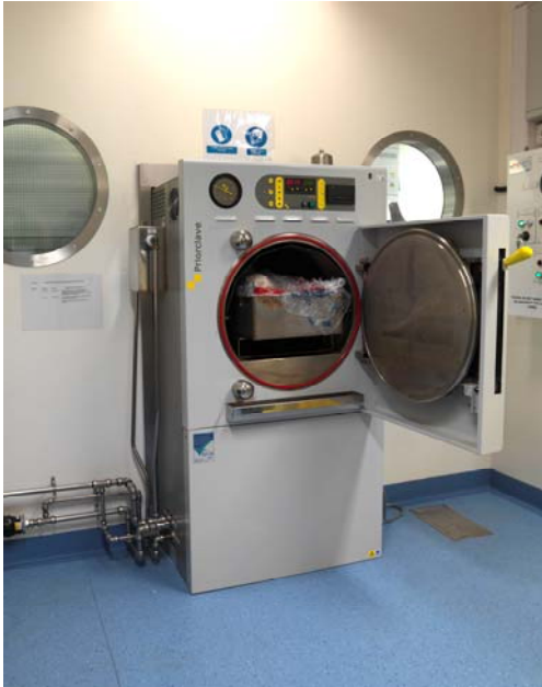
A typical double-door installation within a containment suite in the Royal London Hospital. This view is from the unloading end.
